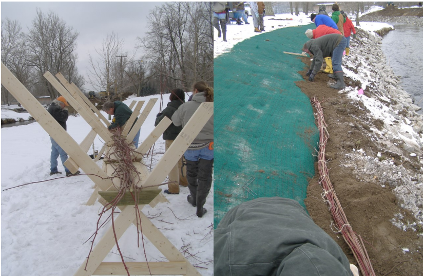
Fascines are first bundled (left) and the laid out and buried along streambank (right).
